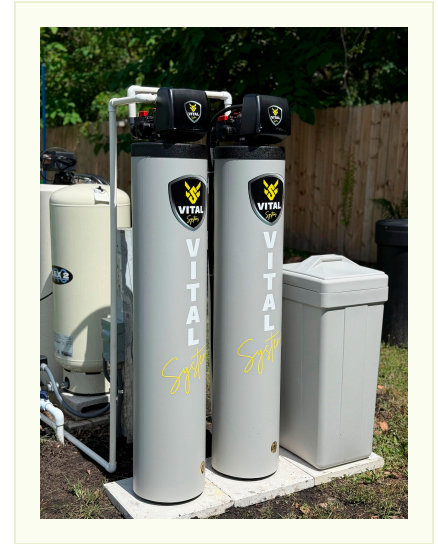
WELL WATER SYSTEM – THREE TANKS
