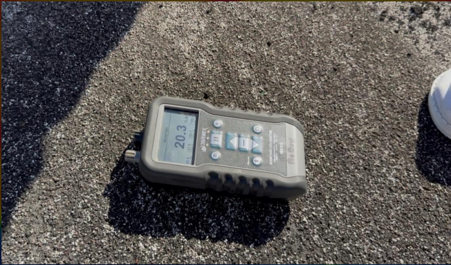
Moisture meters confirm the presence of water inside roofing materials and insulation.
