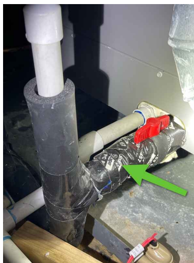
Primary condensate drain line
