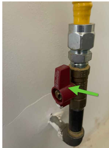
Gas shut off valve
