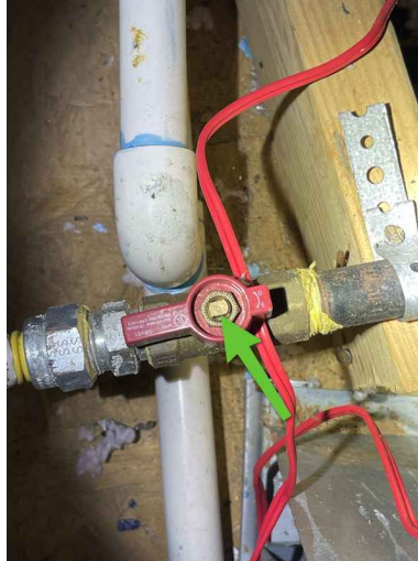
Gas shut off valve
