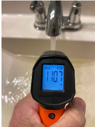
Photo(s) of 1st water heater: Natural Gas, 40-Gallon, Age: 5-10 Years
