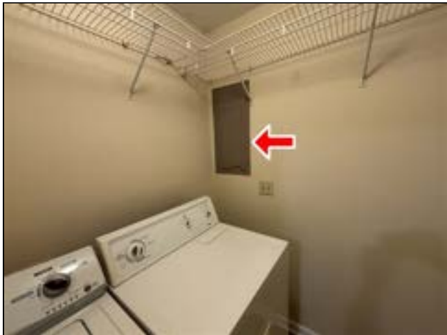
7.1 Item 3 (Picture) The main panel could not be safely accessed due to the laundry machines (we do not move large items or appliances). Be advised a 36" clearance is needed in order to safely remove a panel cover. I recommend having a qualified electrician evaluate further when safe access can be obtained
