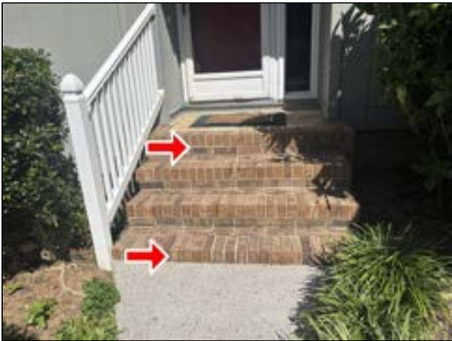
2.3 Item 2 (Picture) Be advised that uneven risers are a potential trip hazard. Correction is recommended for safety.
