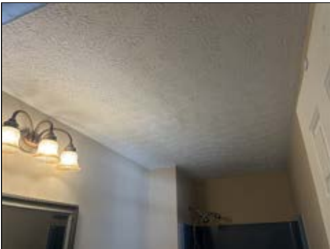
9.4 Item 2 (Picture) Be advised there is no exhaust fan in the hall bathroom. Be sure to open a window when bathing/showering to ventilate the moist humid air to the exterior. A powered fan can also be installed.
