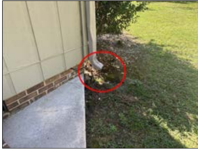
1.3 Item 3 (Picture) The addition of downspout extensions is recommended to divert water away from the home and foundation.
