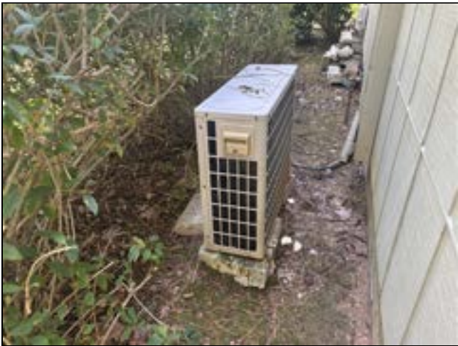
8.8 Item 5 (Picture) HVAC reference
