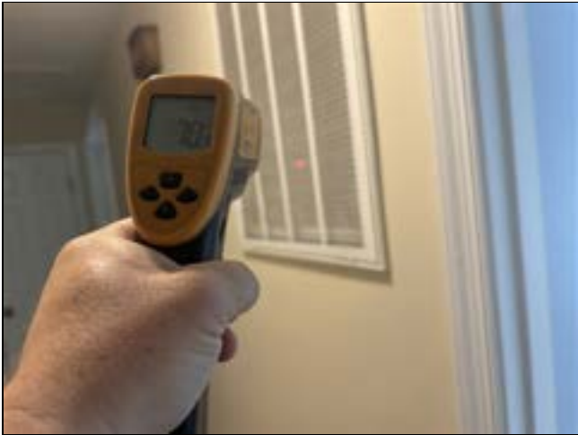
8.9 Item 1 (Picture) A 14° differential was observed during cooling mode
