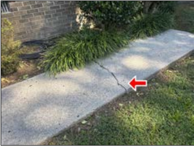
2.4 Item 4 (Picture) I recommend repairing any superficial cracking as desired and/or monitor periodically
