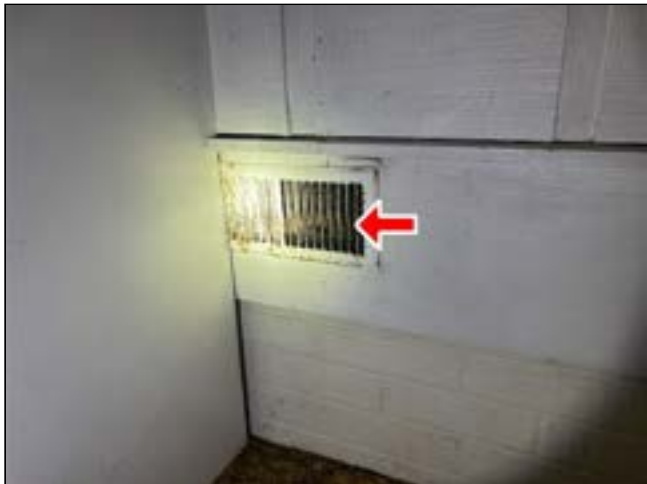
8.3 Item 3 (Picture) view of subject register from inside great room
