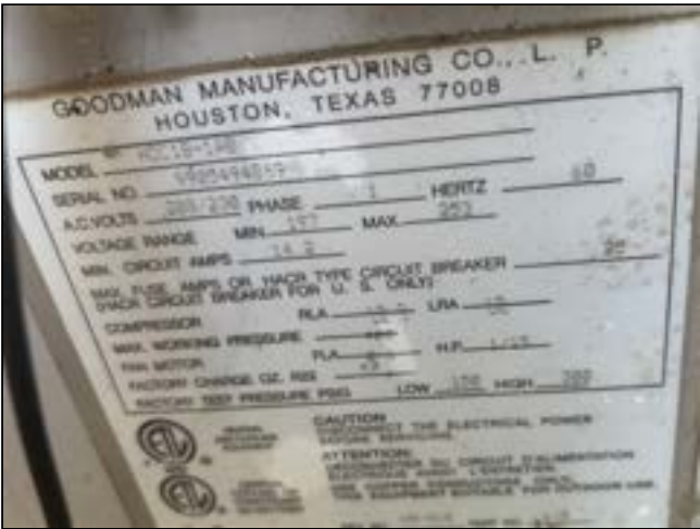
8.8 Item 6 (Picture) HVAC reference
