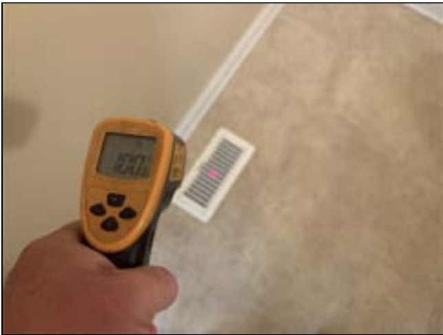
8.1 Item 1 (Picture) temp reading at register during heating mode
