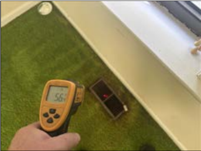
8.9 Item 2 (Picture) A 14° differential was observed during cooling mode
