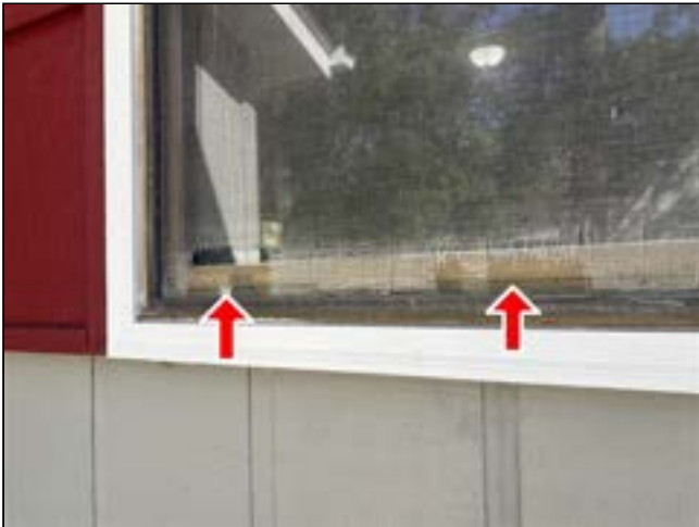
2.2 Item 6 (Picture) Some screens are installed and some are not, and there is minor damage in areas. These are not required so I recommend repair or replace as desired
