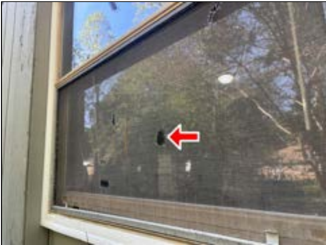
2.2 Item 5 (Picture) Some screens are installed and some are not, and there is minor damage in areas. These are not required so I recommend repair or replace as desired
