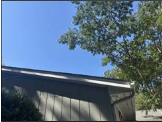
2.4 Item 3 (Picture) It is recommended that the tree limbs in contact with or hanging near the roof be trimmed to help prevent damage, debris, pests from gaining access, etc.
