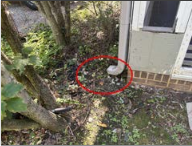
1.3 Item 2 (Picture) The addition of downspout extensions is recommended to divert water away from the home and foundation.
