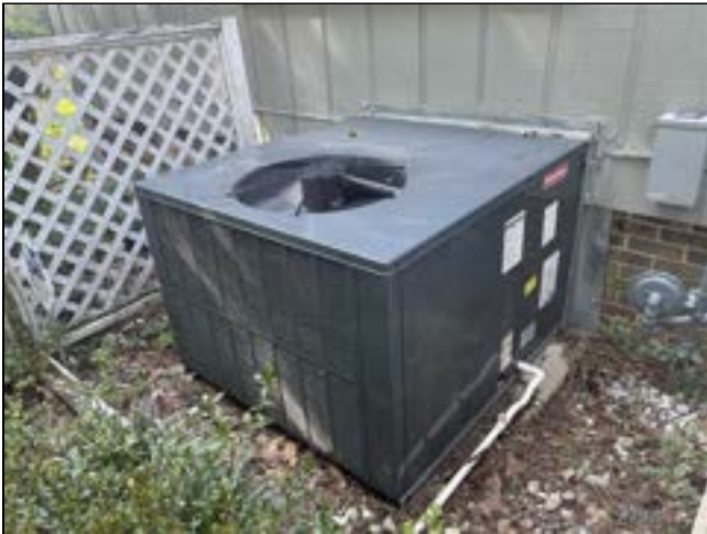
8.8 Item 3 (Picture) HVAC reference
