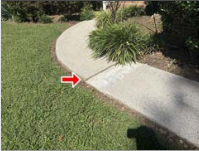
2.4 Item 5 (Picture) Be aware of potential trip hazards at the walkway(s). Correction is recommended for safety
