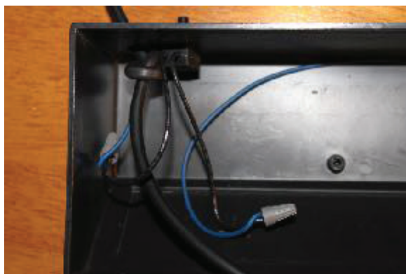
Knot in power cable and switch with wire connectors
