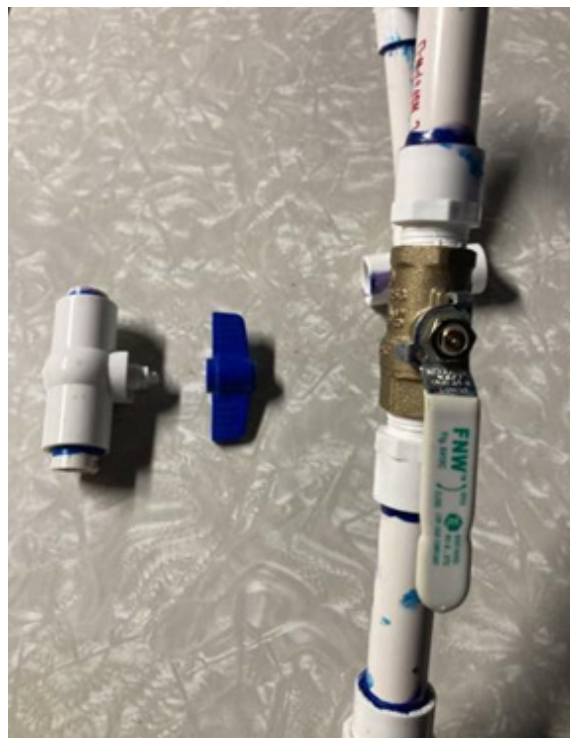
Broken PVC Ball Valve on Left
