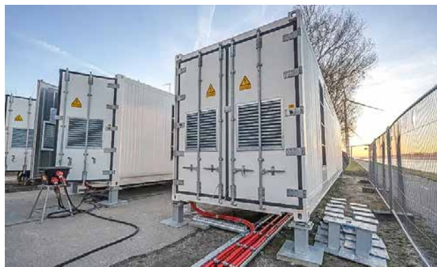
Industrial battery installation
