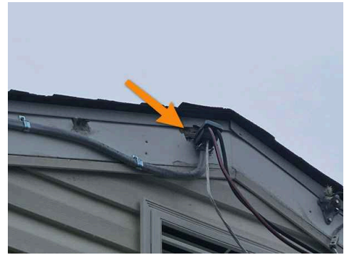
Exposed wood behind the metal flashing
