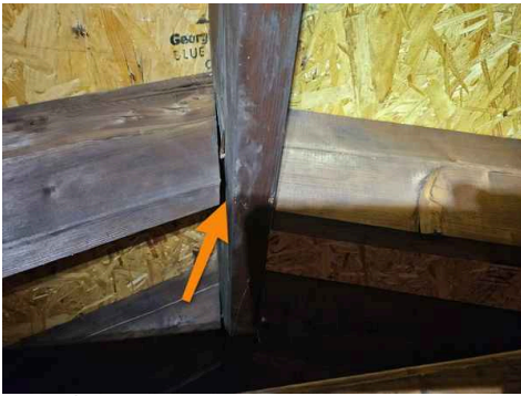
All rafter appeared to be separating from the ridge beam. Recommend installed rafter ties to prevent more movement and separation.
