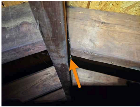
All rafter appeared to be separating from the ridge beam. Recommend installed rafter ties to prevent more movement and separation.
