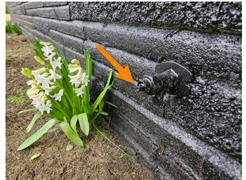
Front - missing handle
