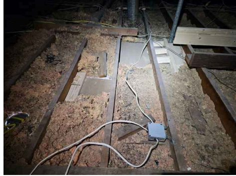
Blown in insulation appeared to be compressed and inadequate throughout the entire attic.
