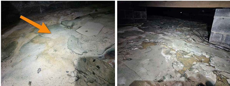
Asphalt material used in which it had dried and became brittle. Recommend having a waterproofing company remove the old vapor barrier and install new 6 mil poly vapor barrier.
