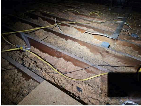
Blown in insulation appeared to be compressed and inadequate throughout the entire attic.
