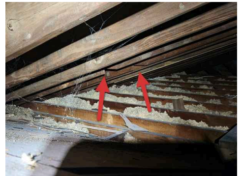
Appears the cut rafters have not been repaired.
