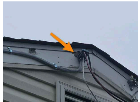
Exposed wood behind the metal flashing
