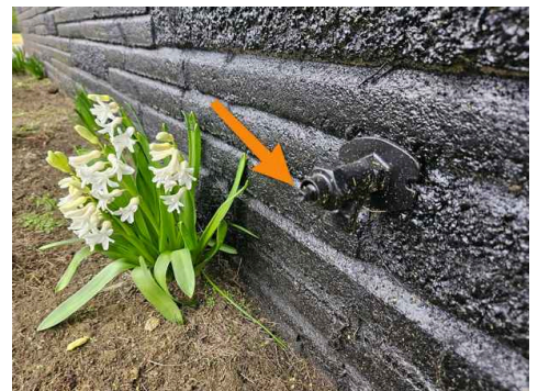
Front - missing handle
