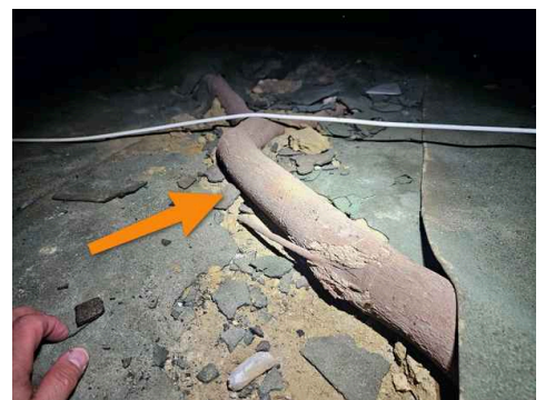
There were roots throughout the crawlspace from the old trees that have been removed around the perimeter of the house.
