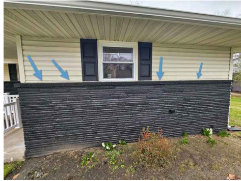
Front - Along the front edge where the vinyl siding meets the stone veneer.
