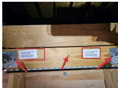
Improper fasteners used to install the folding attic ladder
