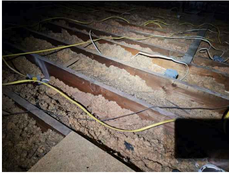
Blown in insulation appeared to be compressed and inadequate throughout the entire attic.
