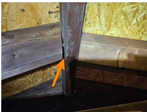
All rafter appeared to be separating from the ridge beam. Recommend installed rafter ties to prevent more movement and separation.
