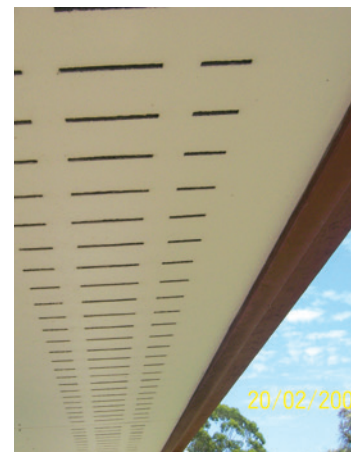
Slotted hardi flex soffit sheeting
