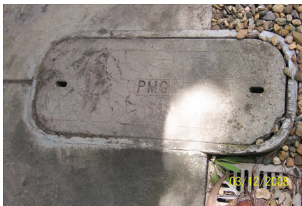
Moulded telecommunications pit
