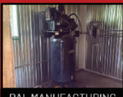
PAL MANUFACTURING AIR COMPRESSOR
