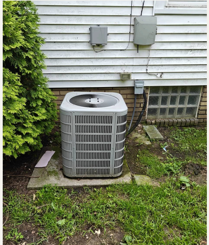
Central air condenser on pad with dedicated circuit
