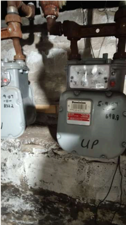
Two gas meters, marked for the lower and upper units
