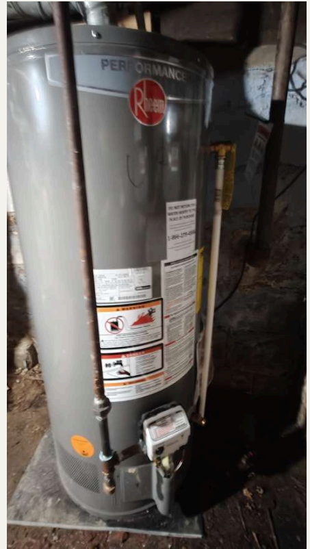
Gas water heater, upper unit
