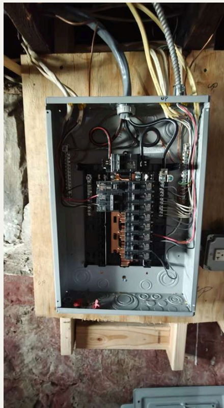
Breaker panel, cover off at the walkthrough
