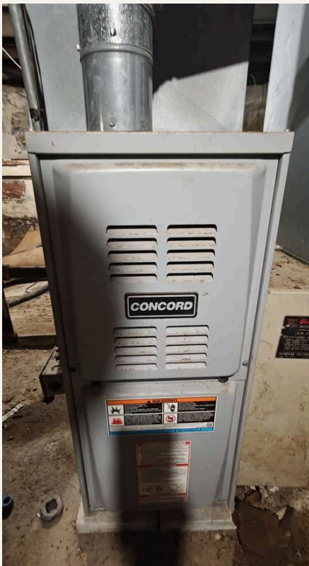
Concord gas forced-air furnace
