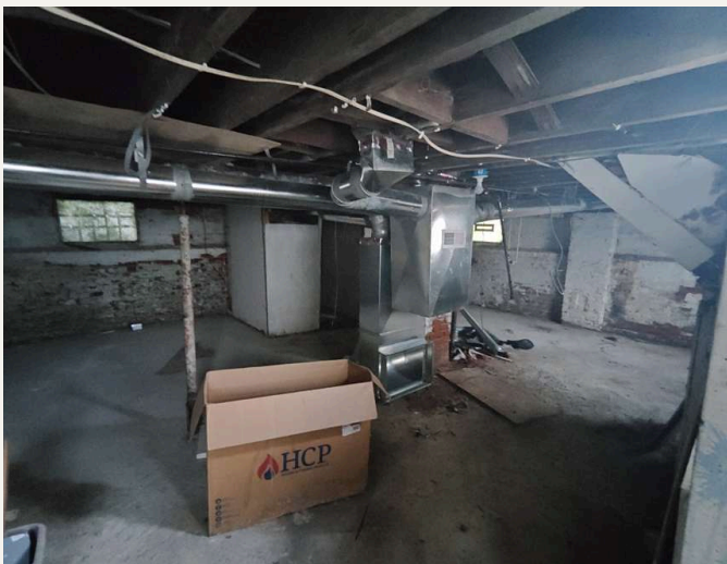
Basement, furnace supply trunk
