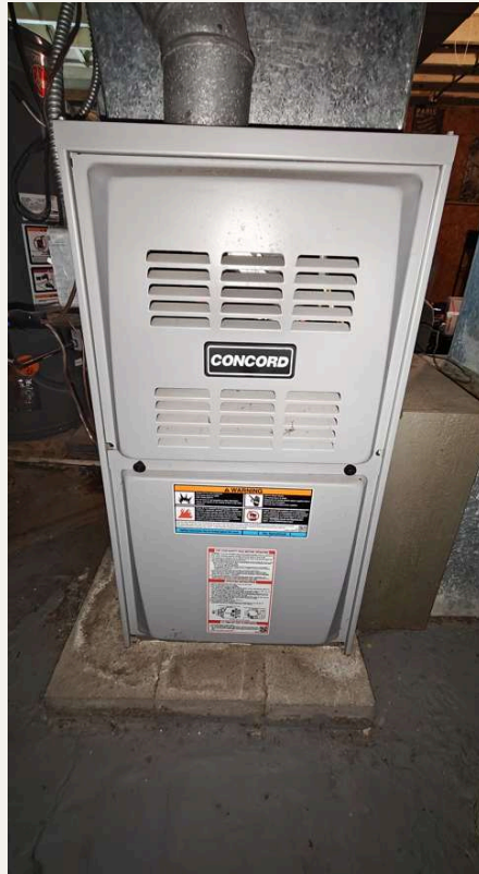
Gas forced-air furnace
