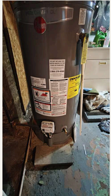
Gas water heater
