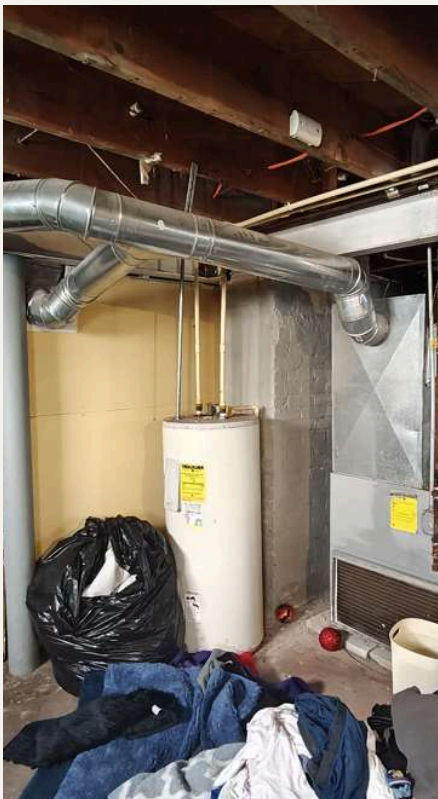
Basement, gas furnace and electric water heater
