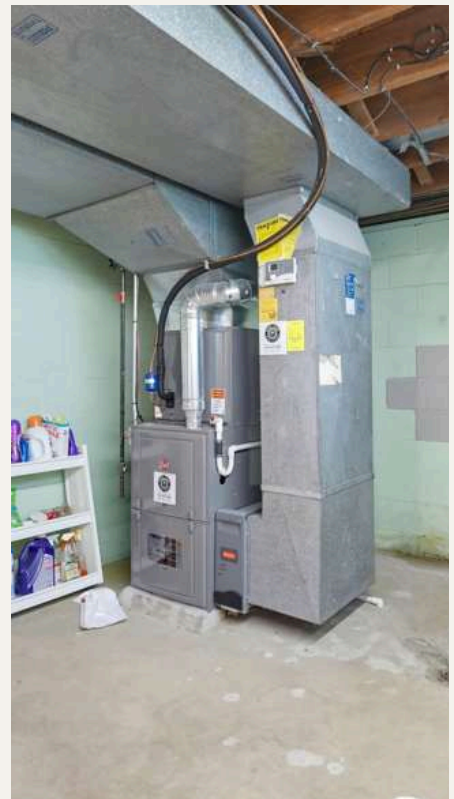
Furnace and mechanicals
