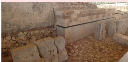
Stones of the Late Bronze Age palace at Hazor, cracked by the fire that burned the city. A modern roof now shelters them. Photo Bukvoed, CC BY 4.0.
