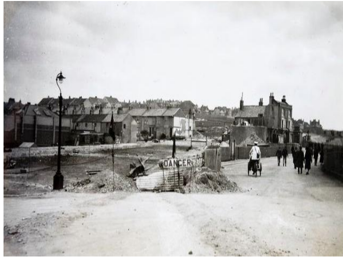
Work in progress on Marine Drive (left) looking east from Black Rock. The road cut straight through the houses in Rifle Butt Road. The old coast road (right) still led to the Abergavenny Arms, the only remaining building at the cliff edge.
