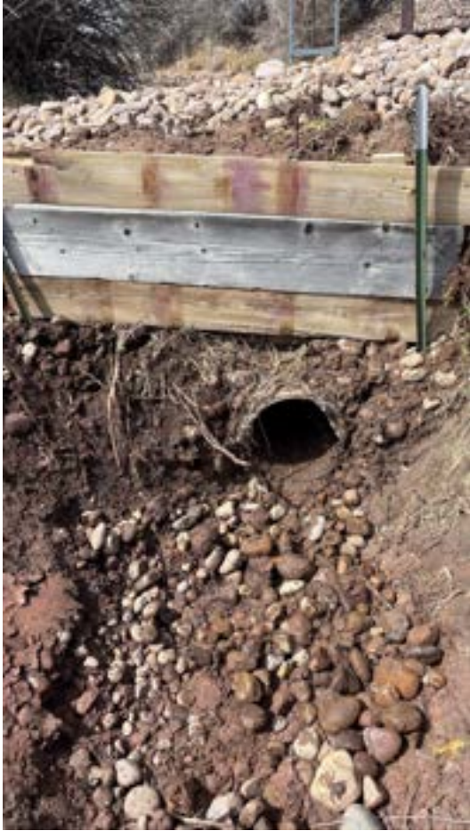
Headgate #7 flow fixed with boards to reduce rock moving into ditch
