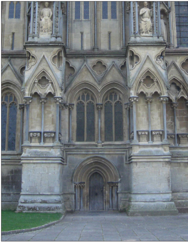
The north-west side-door and its windows directly above which are out of alignment with the door as well as the architecture above the windows....
