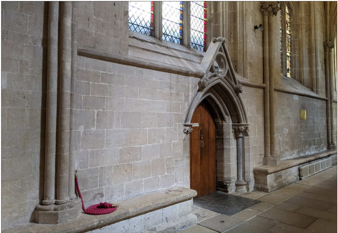
ABOVE - The front door of the sacristy is positioned at the golden section of its bay
