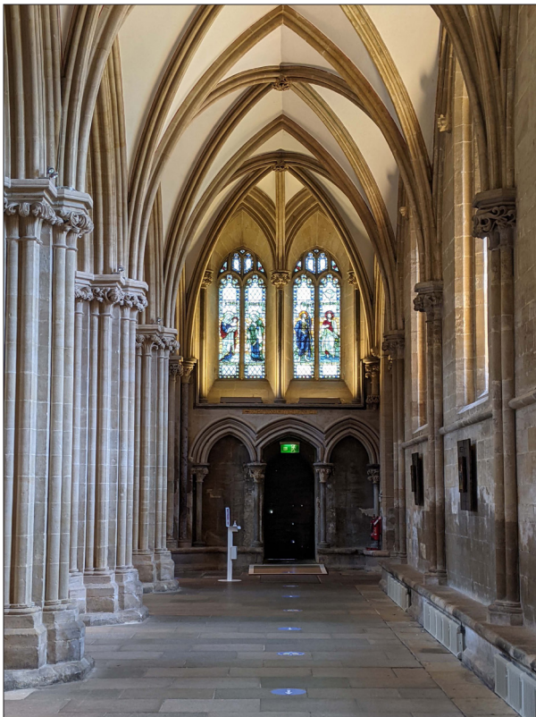
Looking at the north-west door from the inside, its misalignment in relation to the windows is visible. But the windows can be recognised as being in alignment with the central axis of the side aisle as seen within the vault.
