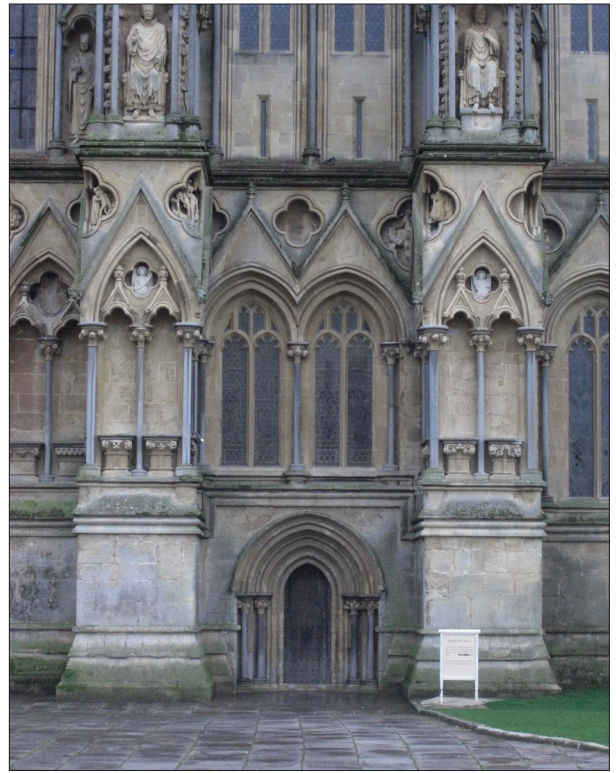
....the inverse equivalent misalignment occurs with south-west side-door
