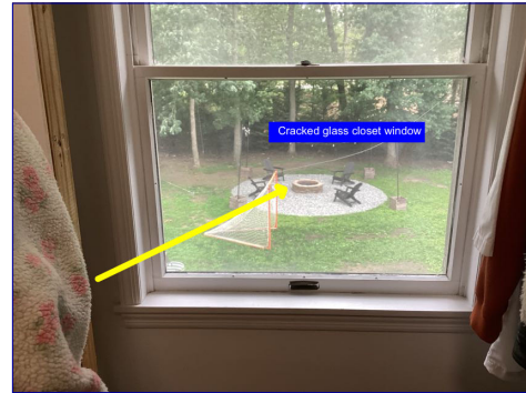
CRACKED GLASS IN MASTER CLOSET
