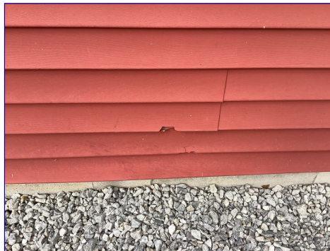
damaged siding in several exterior locations
