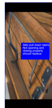
attic stairs in garage should be replaced not working properly
