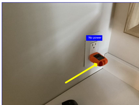
NO POWER TO THIS OUTLET
