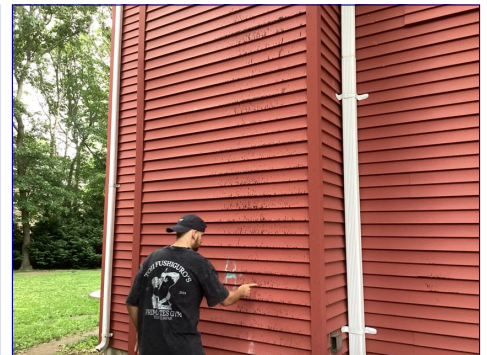
tar on siding
